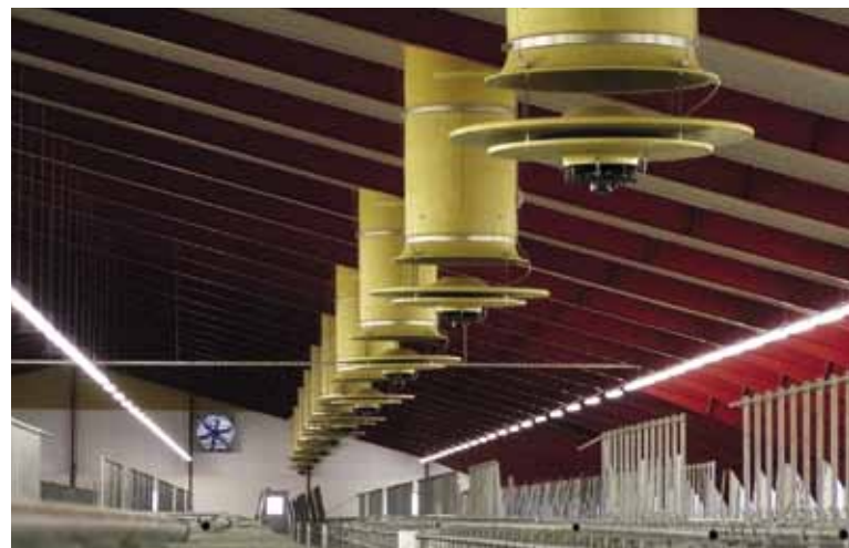
Air Inlet / Recirculation Chimney
