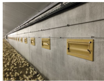
TPI ventilation in a poultry house
