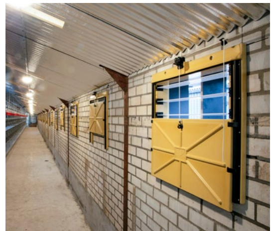
TPI Polytechnik's OmniFlux inlets installed in Dutch poultry farm
