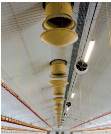
TPI Polytechniek – ventilation in a pig house
